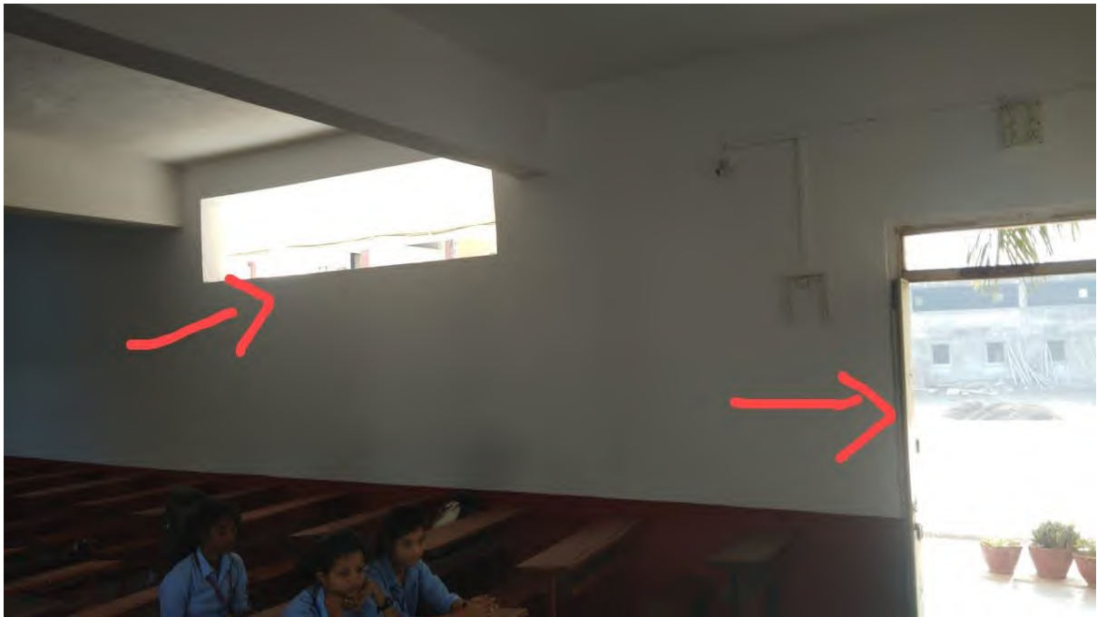
Photo 18 Classrooms of the college Campus are Well Ventilated, with a very good Window Floor ratio.
